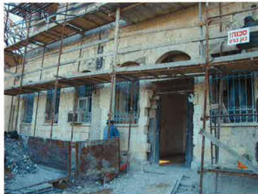
Be'er Sheva Project: damage done by rising salts from ground and application of modern cement plasters.
